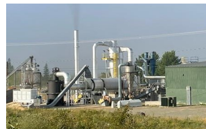
CoalSwitch® Reference plant – Sept 2022
