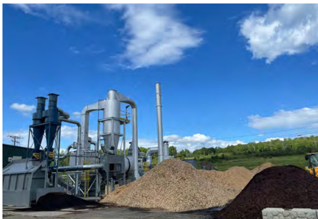
CoalSwitch® production at Ashland, July 2021.
