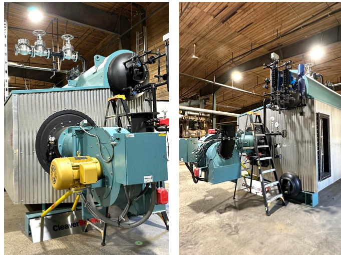
Ashland factory facility equipment – July 2023
